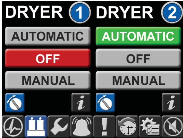
Figure A.1 Main Screen - Dryer Operation
